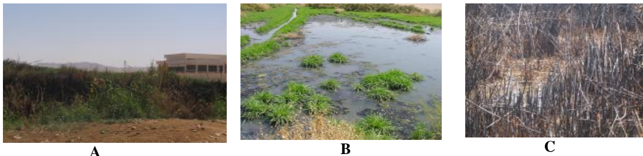
Fig. 2 A: Deterioration of properties at the Qena sewage water treatment plant. B, C: Seepage of wastewater and formation of ponds.
